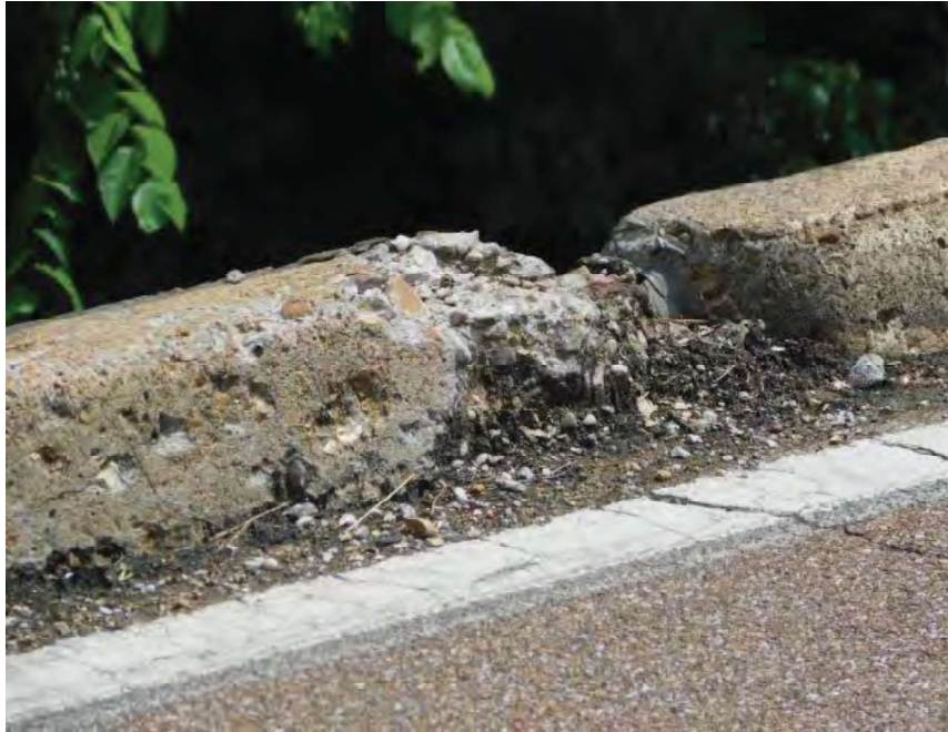
LEFT SIDE SPAN 1 CURB SPALLED TO STEEL
