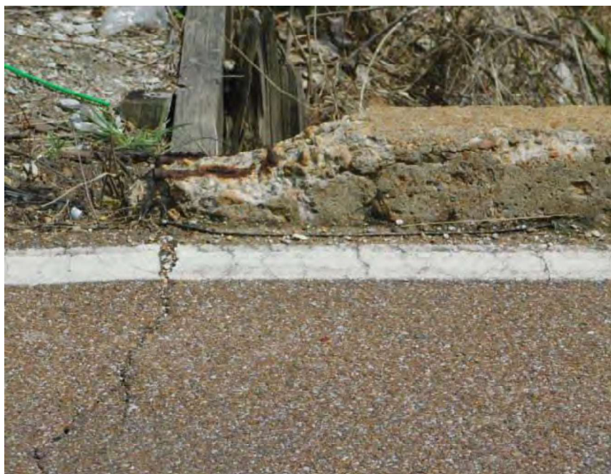
LEFT SIDE SPAN 1 CURB SPALLED TO STEEL
